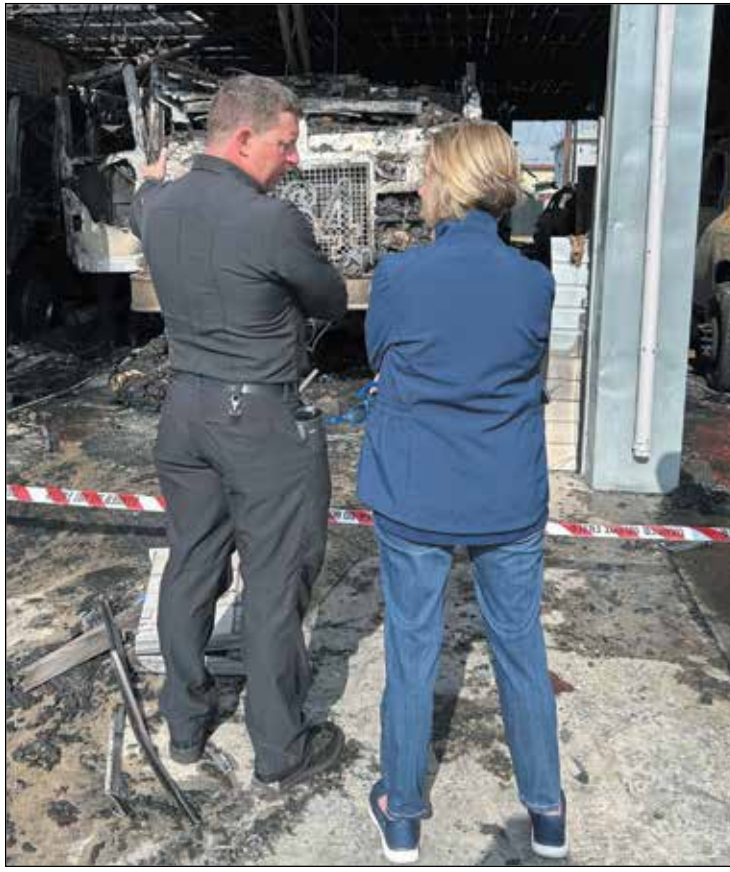
Janice Hahn visits the damage fire station in Huntington Park on Wednesday.
