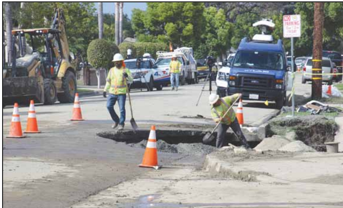
A traffic collision Saturday night resulted in a sinkhole on Rives Avenue and Brunache Street, knocking out electricity and water service to neighborhood residents. Photo by Alex Dominguez
