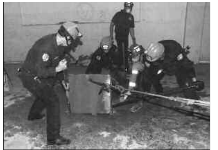
The Downey Fire Department hosted a multi-jurisdictional search and rescue drill July 23 at the soon-to-be demolished Verizon building on 2nd Street. Search and rescue teams from Downey, Santa Fe Springs, Vernon and Compton participated in an earthquake scenario drill that required rescue of victims under concrete floors. Each team was required to cut out a section of concrete floor without the floor falling onto the victims.
