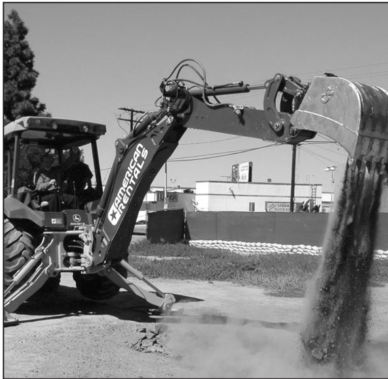
Desert Reign Assembly of God's new sanctuary and offices should be complete in eight to nine months, church officials said.
