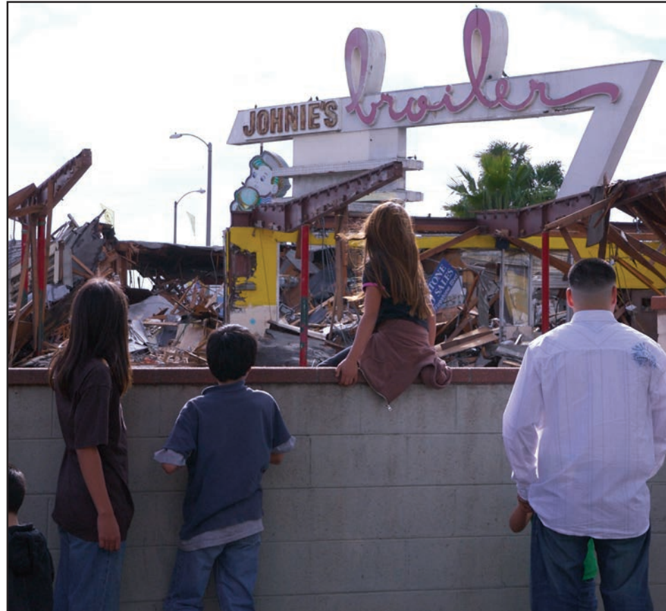
Passerbys look over what remains of Johnnie's Broiler, which was nearly completely demolished last January. The tenant of the property was charged with five misdemeanor counts this week. Photo by James Quick III/Brooks Institute of Photography
