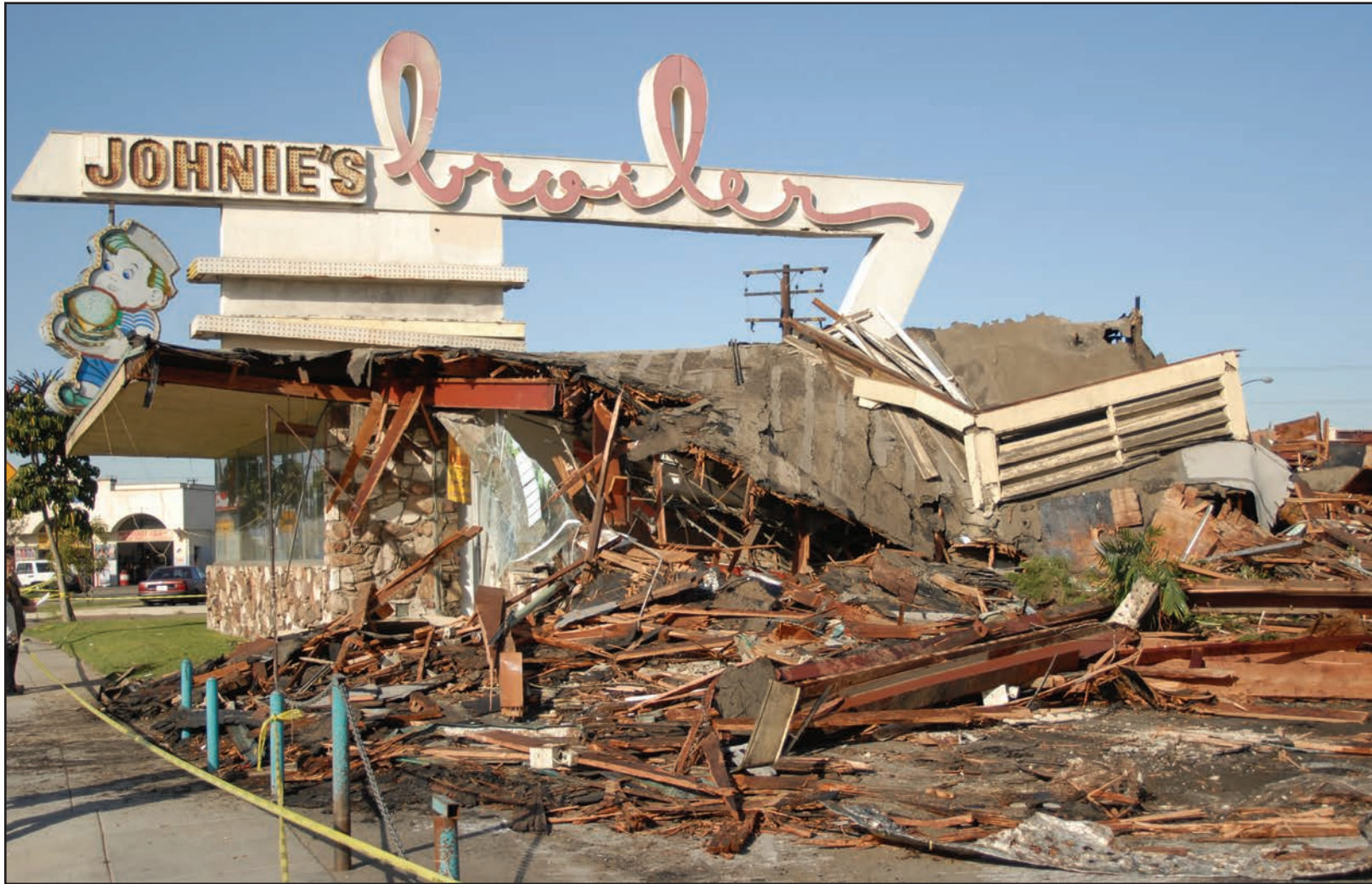
Demolition on Johnie's Broiler started Sunday afternoon and continued until Downey police stopped it some two hours later. By then, however, the damage had been done. Photo by Art Montoya
