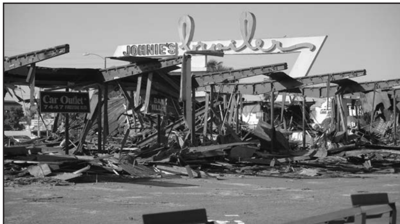
"T" shaped steel frames resting on a reinforced concrete foundation was no match for a bulldozer. Photo by Art Montoya
