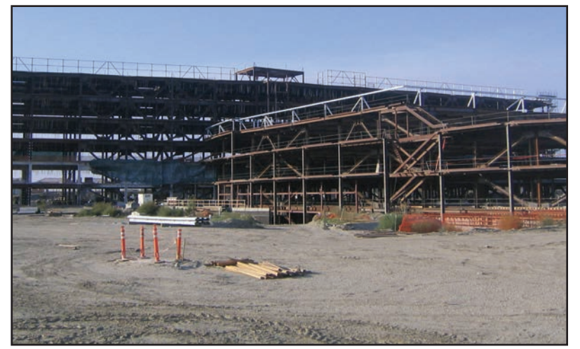
NOT MUCH RIGHT NOW – The dusty construction site on Imperial Highway will soon be home to a new 657,000 square-foot medical complex.
